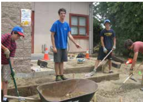
Nick Grabert (in blue) and his fellow Scouts building the new walkway.
